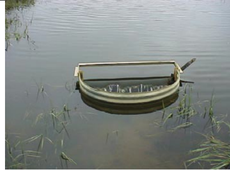
Vertical standpipe with wooden flashboard riser
