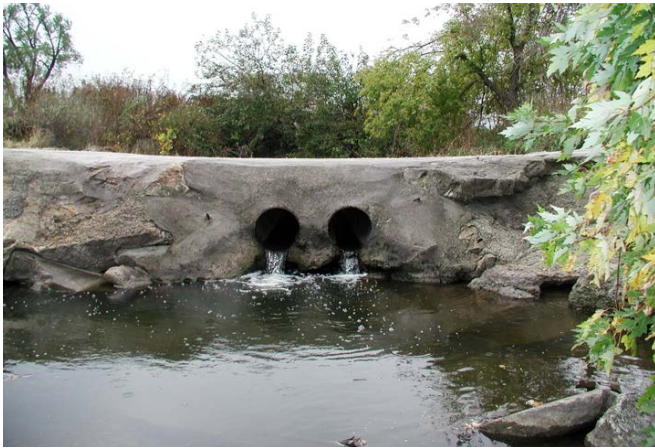
Figure 3. A low water crossing with channel incision or poor design, like this one, creates a barrier to fish and other aquatic organisms.
